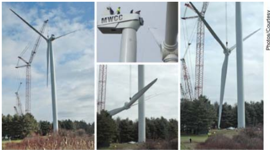
WINDED: Mount Wachusett Community College of Gardner recently completed the installation of its first wind turbine. The school is one of several in Central Massachusetts to take on green projects in the last year.
