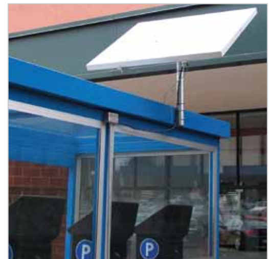
The photovoltaic array Ameresco designed and supplied to Amano McGann to power the Norwalk Parking Authority's parking meter shelter.
