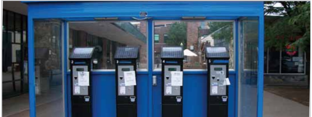
Of the 13 photovoltaic-powered parking meter shelters constructed, this was the only shelter to boast multiple meters and arrays. Above each pay meter is a photovoltaic module.
