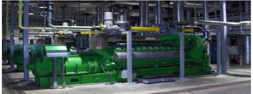
At the Southside Wastewater Treatment Plant in Dallas, Ameresco designed a cogeneration facility that utilizes the biogas to feed three generators. The heat captured from the engines produces hot water, which is utilized by the digesters.
