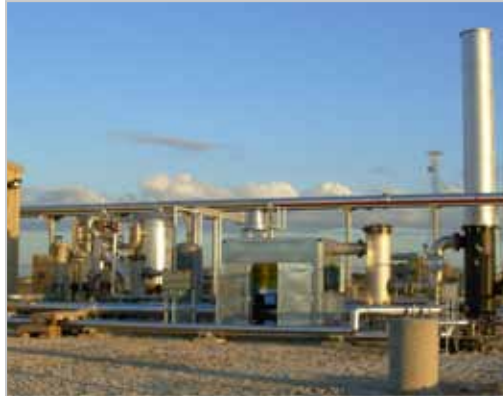
The facility provides a guaranteed minimum amount of hot water for heating the round-the-clock operations of the digester vessels and boilers, and a minimum amount of electricity.
