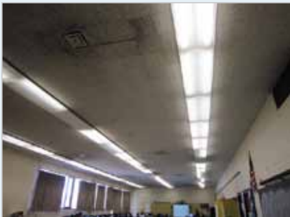
Ameresco will replace old inefficient lighting, which not only increase energy savings but also improve aesthetics.
