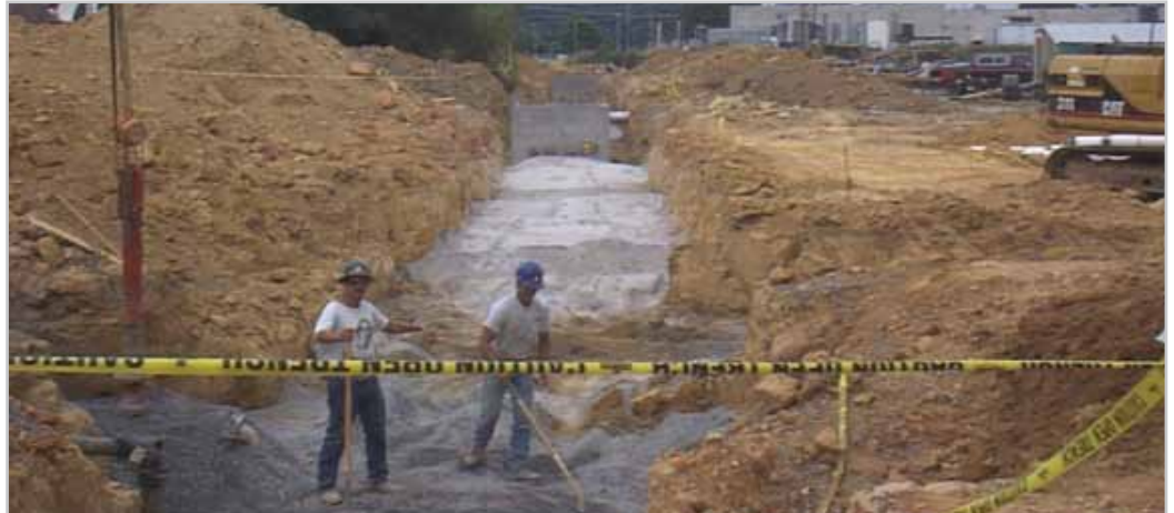
The construction crew lays the groundwork for the underground steam distribution pipeline.
