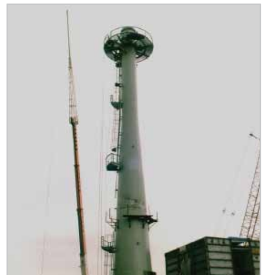
The exhaust from the wood chips being burnt is captured in this stack.
