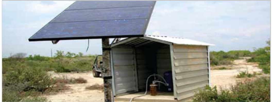
Ameresco helped Burts Ranch achieve a solution for its water needs by designing a solar-powered pump that will draw water to the ranch and storage tank.
