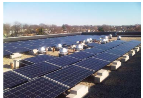
The Cambridge Housing Authority installed a 46 kW grid tie solar PV system.
