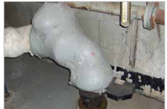
From the outdated centralized and leaking steam heating systems, the CHA constantly faced costly maintenance problems prior to the EPC work.
