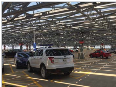
Ameresco replaced 7,743 metal halide light fixtures in 4 parking ramps to energy-saving LED technology.
