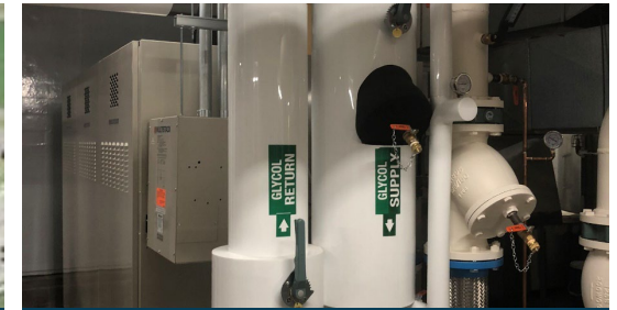
LOW TEMP HEAT PUMP PLANT
