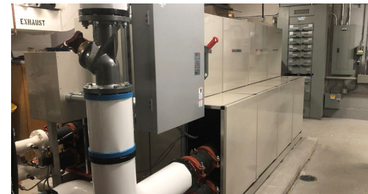
HIGH TEMP HEAT PUMP PLANT
