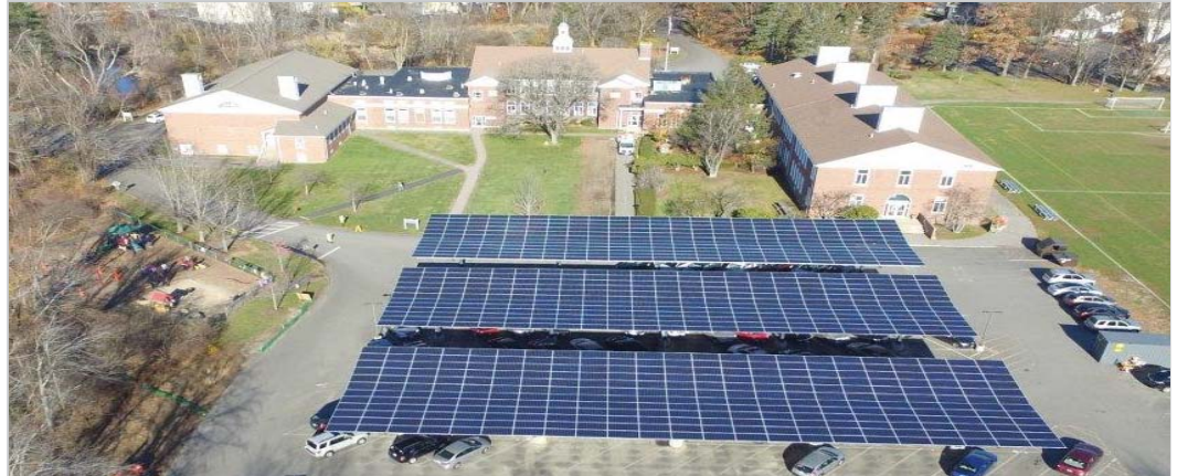
Solar parking lot canopy.
