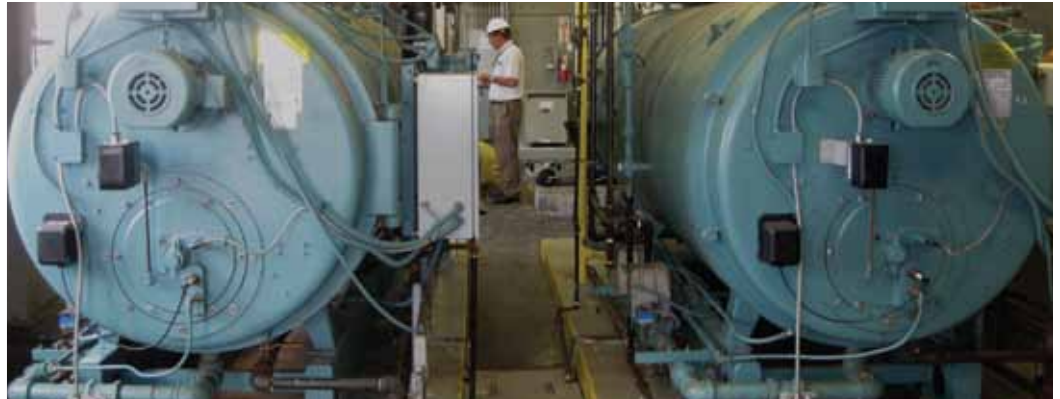
Ameresco reduced Tobyhanna's emissions by converting the primary heating system fuel from coal to natural gas. Emissions were cut by 60 percent.
