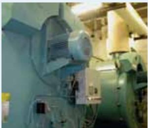
Two of the new decentralized gas-fired boiler plants at Tobyhanna installed to replace a coal-fired boiler plant.
