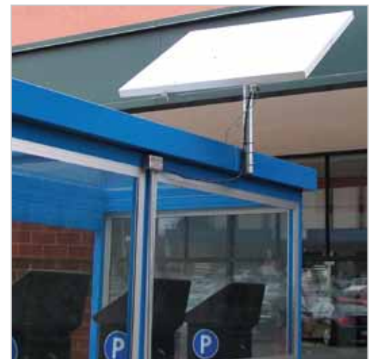
The photovoltaic array Ameresco designed and supplied to Amano McGann to power the Norwalk Parking Authority's parking meter shelter.
