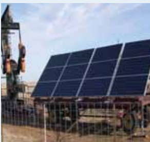
The pump jack pictured is connected to a down-hole cylinder at a depth of approximately 7,500 feet.
