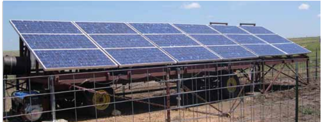
The solar array was expanded from the 12 modules to a total of 18 modules, as pictured. It has an output of 3150Wp. (All photos courtesy of the R & A Moore, Inc.)
