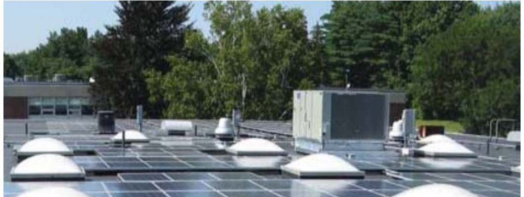
The rooftop of the Rupert Nock Middle School and Edward G. Molin Upper Elementary School features a solar array that transmits data via the Internet to the science classrooms for the students to monitor weather and solar conditions.
