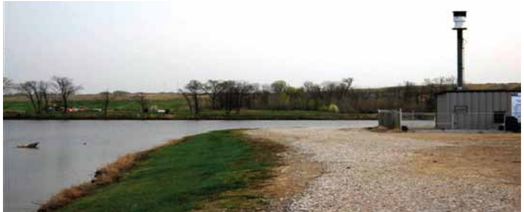
Pipeline for the landfill gas to energy plant was difficult to lay without disrupting traffic and private property, but Ameresco succeeded. The plant became operational in May 2009.
