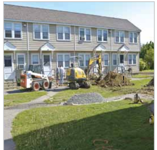
Improvements included the conversion of clothes dryers from electric to natural gas and water conservation measures, such as the installation of low-flow toilets, showerheads, and faucet aerators.
