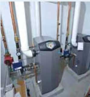
Ameresco decentralized the boiler plant and installed high-efficiency hot water heating, along with new heating baseboards and temperature controls.
